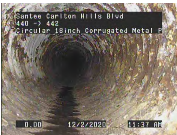
0.00ft Surface Damage Corrosion from 1 o'clock to 10 o'clock, Start
