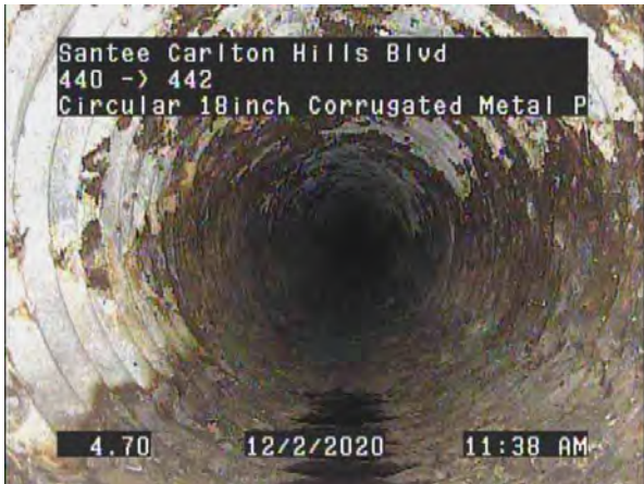
4.70ft Surface Damage Corrosion from 12 o'clock to 12 o'clock, Start
