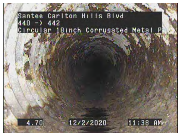
4.70ft Surface Damage Corrosion from 12 o'clock to 12 o'clock, Finish
