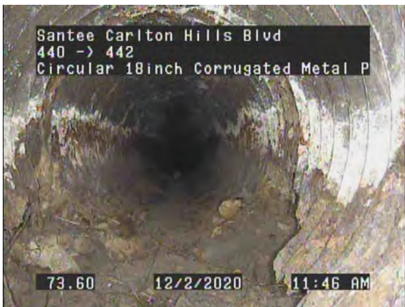
73.60ft Surface Damage Corrosion from 12 o'clock to 12 o'clock, Finish
